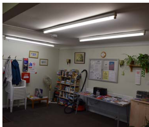
Poor quality fluorescent lighting at Ditchling Gardens
