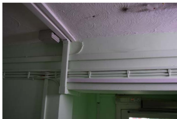
Exposed wiring in corridors is problematic
