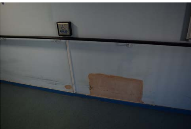
Poor quality paintwork.
