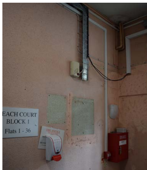
An example of poor quality repair work at Leach Court
