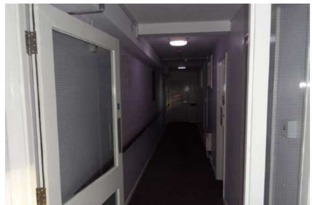
Communal circulation needs redecoration
