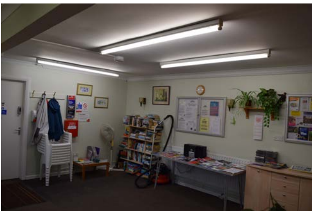
The communal lounge is functional, but could be improved by replacing the lighting
